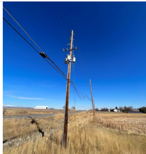
12. Pole-Mounted Transformers (Along 95 th St.)
